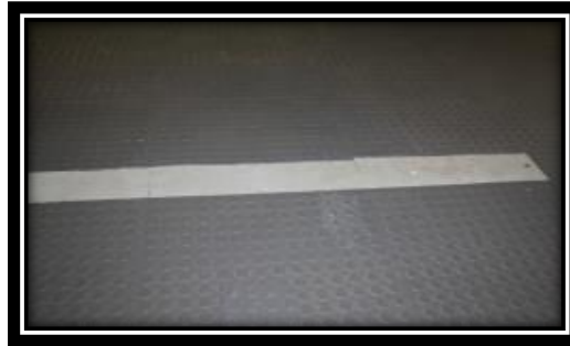
Unsafe floor conditions
